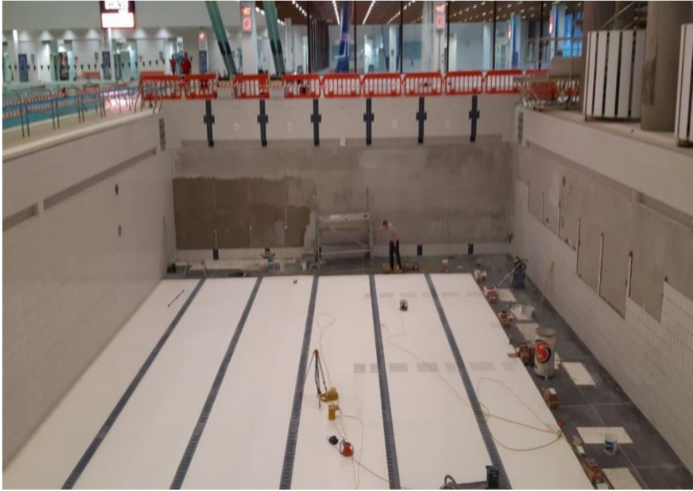
Photograph of Royal Commonwealth Pool during refurbishment (CEC funding contribution to Edinburgh Leisure managed property)
